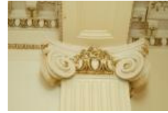
Lead paint in Foyer
